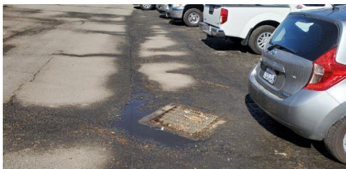
End of Drainage Backflow
