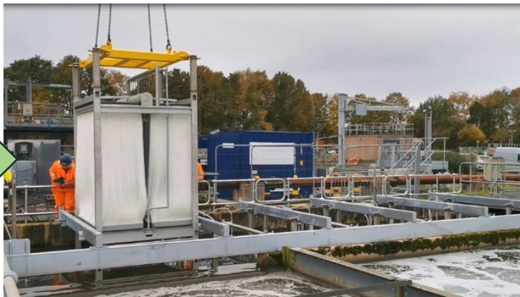
Full-Scale Demonstration of MABR in Existing Aeration Tanks in 2026 (as Part of the Nutrient Management, DP 100078)
